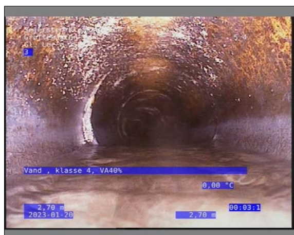
Foto: 3_1_7_20012023_093915_1.JPG 2,7m, Vand , klasse 4 / VA40%
