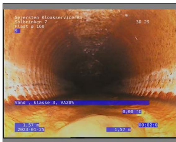
Foto: 18_1_8_25012023_104010_1.JPG 1,57m, Vand, klasse 3 / VA20%
