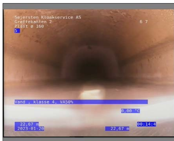
Foto: 4_1_27_20012023_104230_1.JPG 22,67m, Vand , klasse 4 / VA50%
